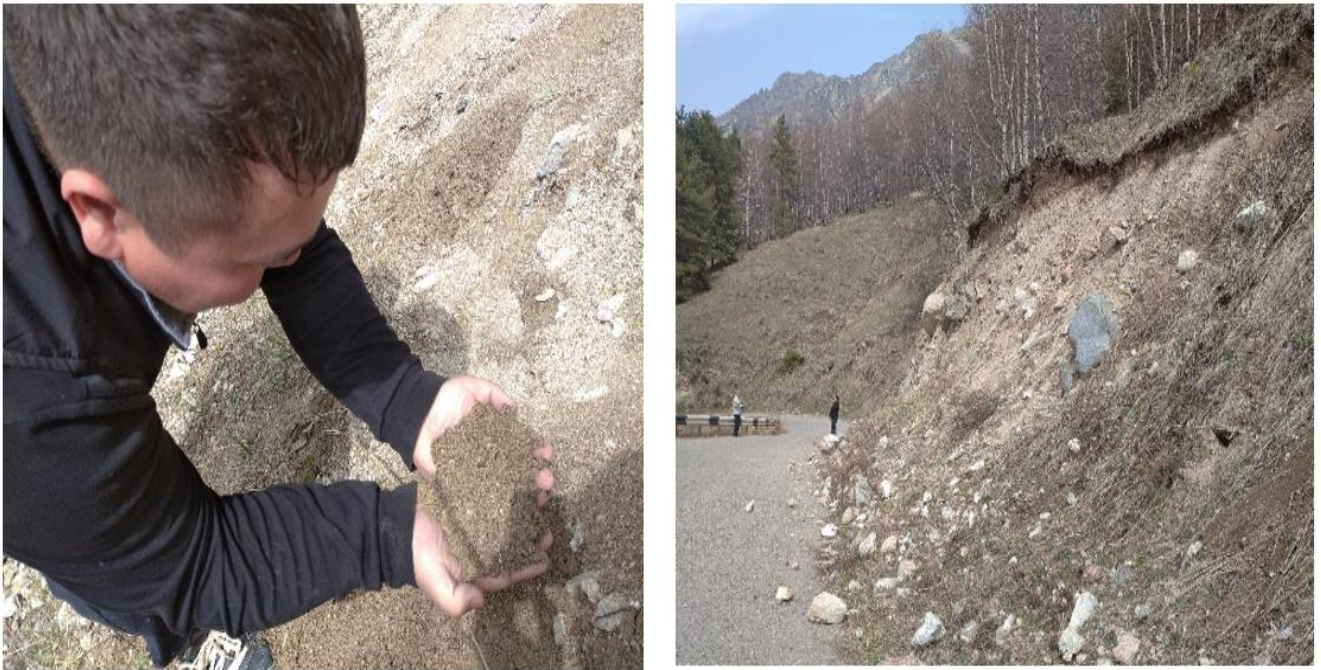
Figure 11. Weak soils of mountain slopes, creating a shear force on the base of the pavement.
